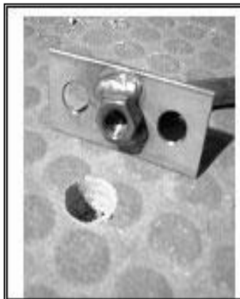
Figure 4 - A pocket has been created for the 1/2" nut that is welded to the bottom of the Floor Plates
